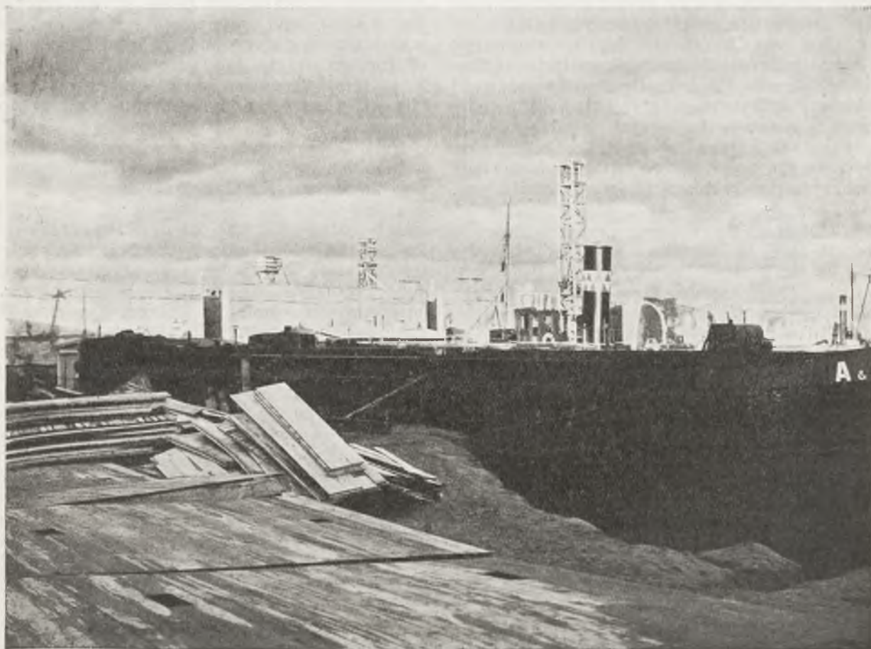
A PORTION OF THE PORT OF GDYNIA, UNDER CONSTRUCTION (PHOT. S. PLATER)
