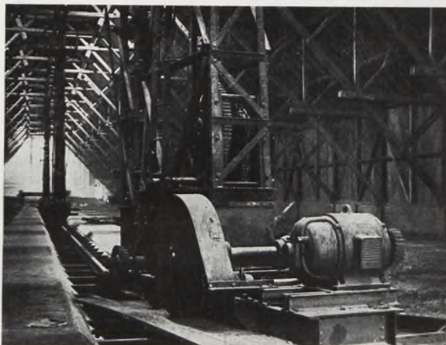
A PORTION OF THE POTASSIUM SALT CONCENTRATING PLANT AT KALUSZ, UNDER CONSTRUCTION (PHOT. S. PLATER)
