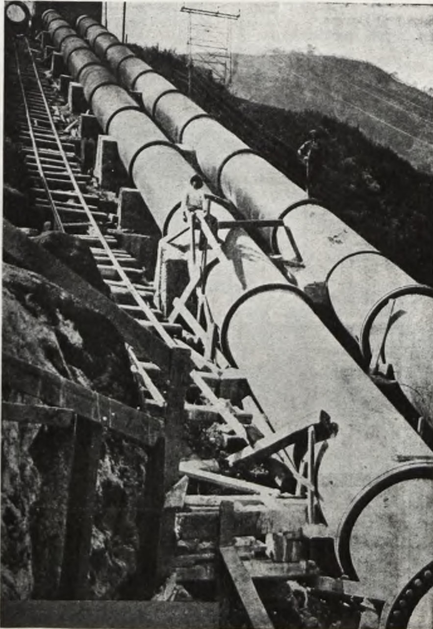
TWO HIGH-PRESSURE WATER MAINS LAID AT HAKONE, JAPAN, BY MESSRS. "FERRUM", KATOWICE
