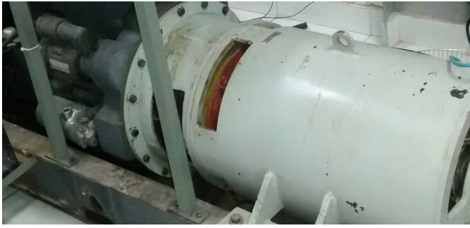
(b) Synchronous Generator
