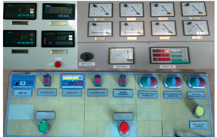
Photo 1. View of an old control room with control and measurement devices
