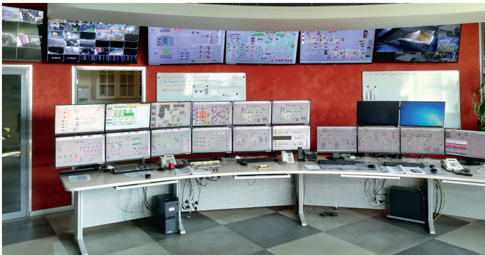
Photo 3. Fragment of a modern DCS MASTER control room with LCD monitors and a touch panel
