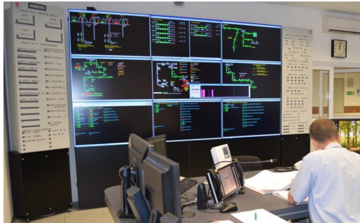
Fig. 4. Tauron's control room [7]
