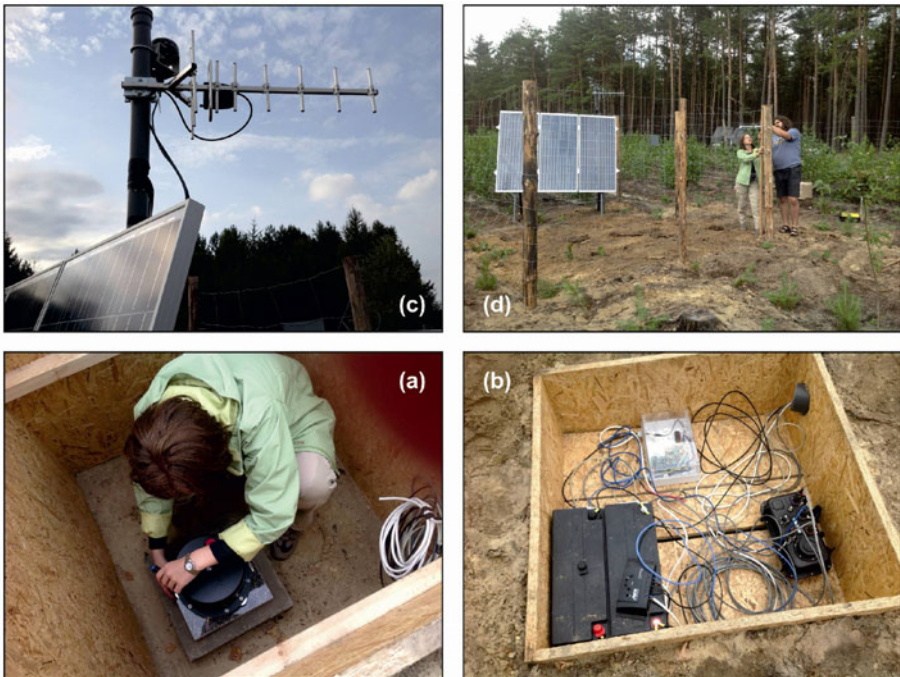
Fig. 4. Installation of the temporary broadband station in northern Poland: (a) Leveling broadband seismometer Reftek 151-120 on the granitic base in the ca. 1 m deep case; (b) Batteries, converter and recorder on the shelf, over the seismometer; (c) Solar panel, GPS and antenna for cell phone connection; (d) Closing the “garden” of seismic station in the forest area (photos taken by M. Grad, June 2013).
