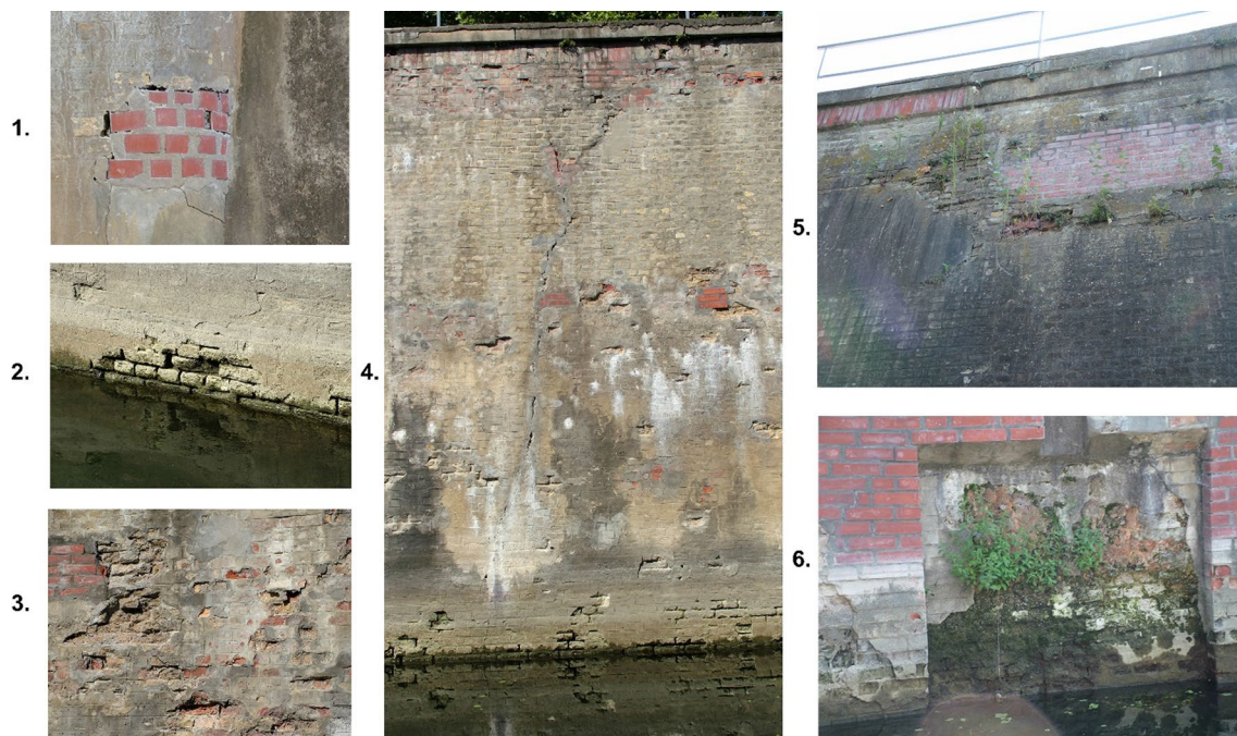
Fig. 3 Recent state of the western wall (1. incompetent repair, 2–3. brick and fugue damages, 4. fault and dissolved mortar, 5–6. wet wall with vegetation)
