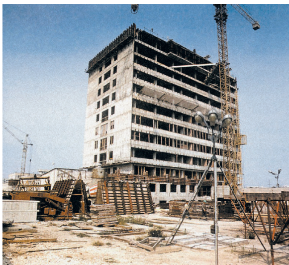
Figure 30. The construction of the new seat of the Institute of Oncology in Ursynów – the scientific building is constructed (from the collections of the editing office of the MSCNRIO)
