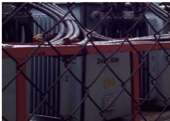
Figure 4. Thermal scanning and actual images of CTU 3 x 250kVA transformer
