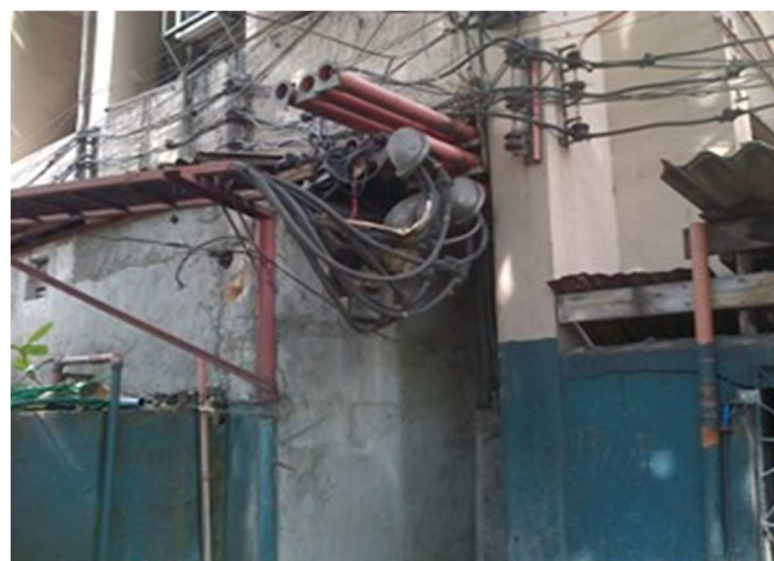
Figure 5. Cable splices from transformer towards main distribution panel
