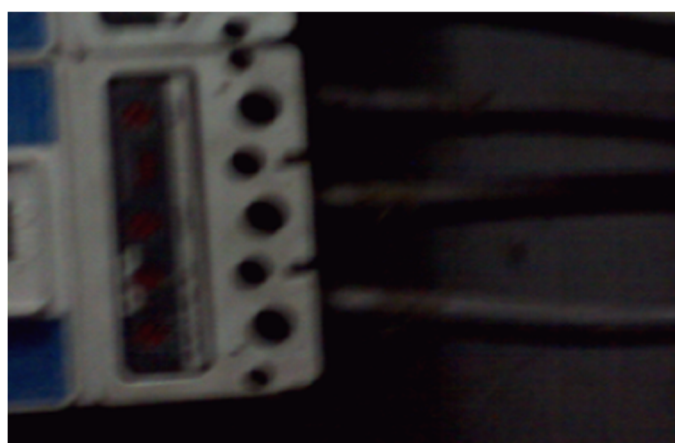
Figure 6. Hot spot at 400 Amperes supplying College of Technology
