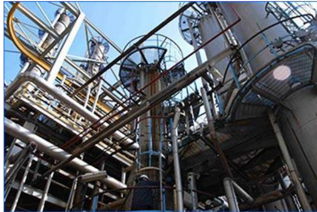
Fig. 2. Technological pipelines Source: udt.gov.pl
