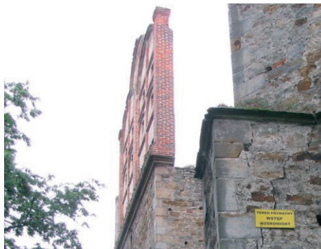
Photo 6. Examples of cracks in a slender attic wall /castle in Drzewica/
