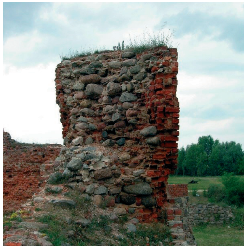
Photo 3. Damages of the "opus emplectum" wall (photographer – Marek Krysiński) /Międzygórz castle/
