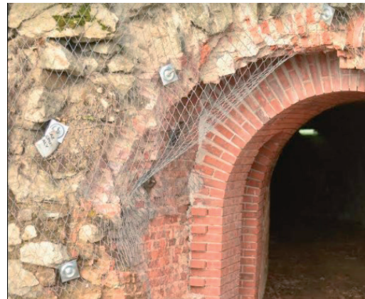
Photo 9. Protection of the damaged wall's face with a steel mesh mounted by the anchors (photographer – Grzegorz Basiński)
