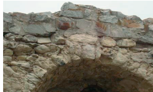
Fig. 21. Addition made of foreign material without the isolation layer. (The castle in Janowiec on the Vistula River)
