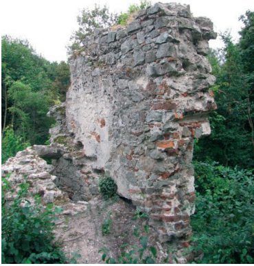
Photo 1. Degradation of the wall due to the environmental factors /Międzygórz castle/
