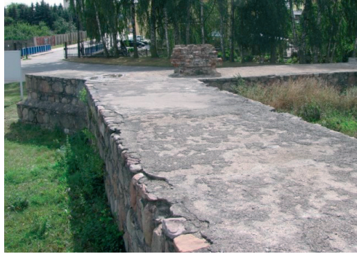
Fig. 25. The crest secured with a layer of cement mortar – without molding. (The castle in Rawa Mazowiecka)
