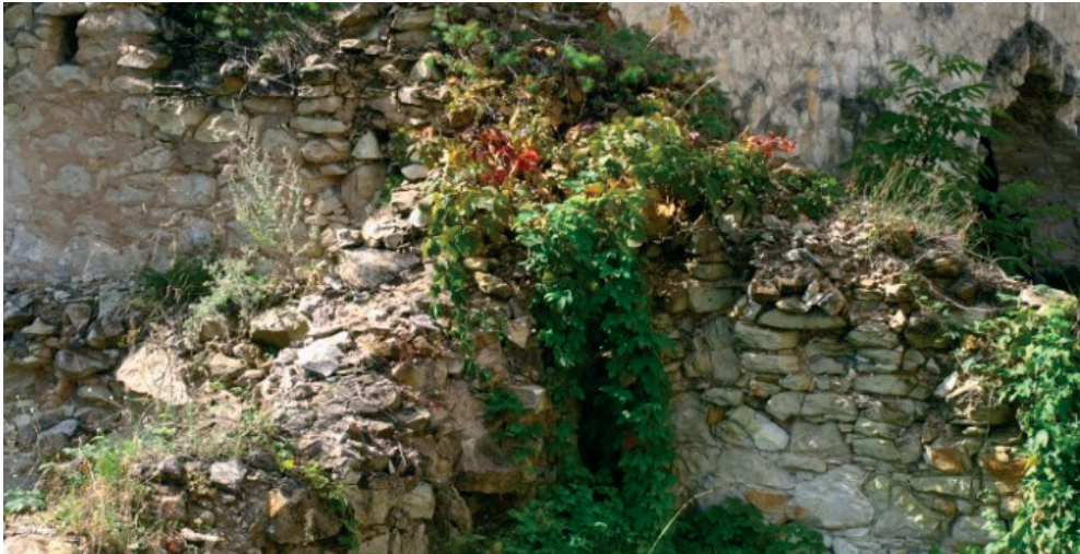
Fig. 16. A significant amount of annuals and perennials causing the degradation of the crown and the loss of legibility of the wall outline (contour).
