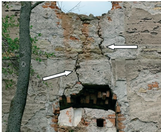
Photo 7. Example of the window head's damage /Panków castle/
