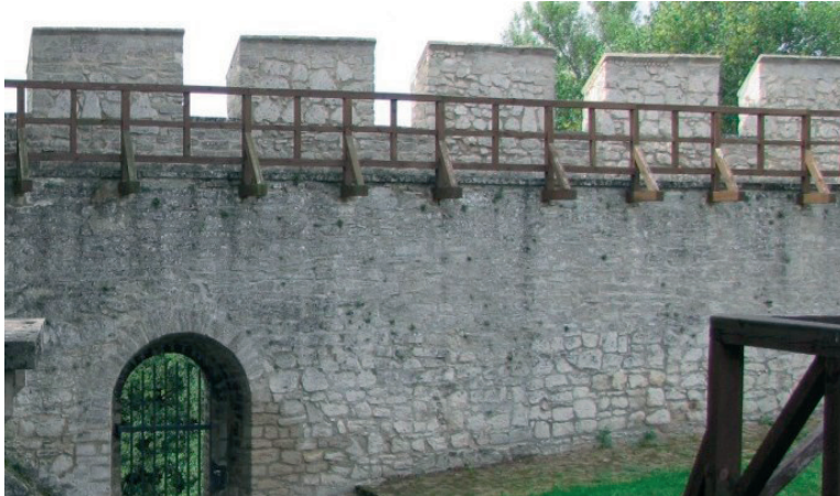
Fig. 19. Reconstruction of substantial fragments of the wall with the material compatible with the historical one)
