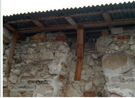
Fig. 33. Securing of the crest and a detail by a wooden construction with corrugated sheet metal (The castle in Janowiec on the Vistula River)
