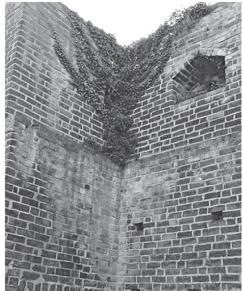
Fig. 2. The development of algae and lichen in the corner of the wall directly under the ivy, which is growing the wall and the crown
