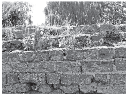
Fig. 10. The expansion of low plants and mosses on the crown of the ceramic brick wall. In the foreground young shrubs are visible
