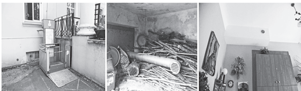
Fig. 4. The secondary solutions aimed at improvement of living conditions and functionality of the building. From left: the elevator beside the main entrance, mechanical installation under the terrace of the garden, ventilation grill inside the building. (Photo: the author)
