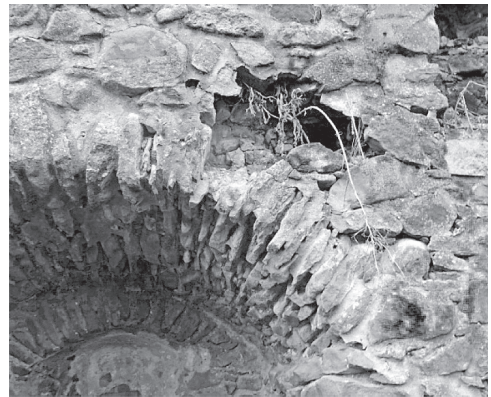
Fig. 8. Damage to the face of the wall associated with the growth of the root system of low vegetation
