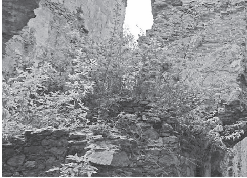
Fig. 13. A fragment of the vault intensely overgrown with shrubs
