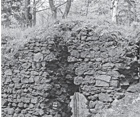
Fig. 11. The low crown of the wall completely overgrown with greenery. The tight layer of humus and greenery prevents evaporation of the moisture retained in the wall
