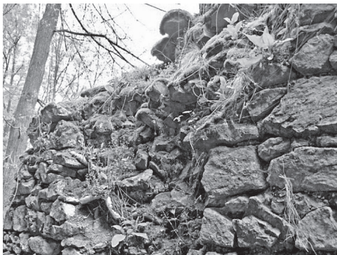
Fig. 9. The crown and the face of the curtain wall planted with a single and perennial vegetation
