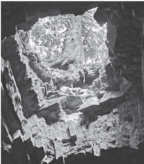
Fig. 17. Vault made of ceramic brick damaged by roots
