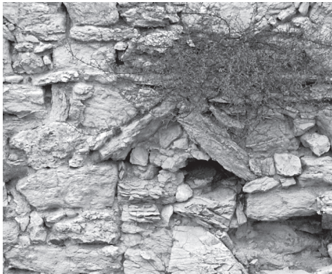
Fig. 7. Photograph of a heavily sunlit southern facade. The development of vegetation in the wall crevices
