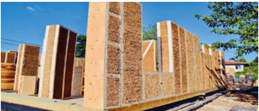
Fig. 3. Walls made of EcoCocon straw panels. Vastu Home – Bulgaria house design, source: www.ecococon.it
