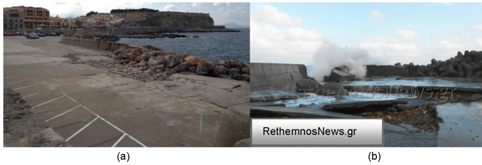
Figure 4 Damages of the base of windward wave breakwater: (a) previous damages, photograph taken on January 4th, 2014; (b) new damages after structural repairs, photograph taken on January 14th, 2015.
