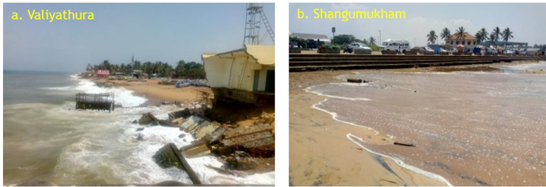
Figure 9 Field photographs of Valiyathura – Shangumukham stretch during the event on 18 March 2019.
